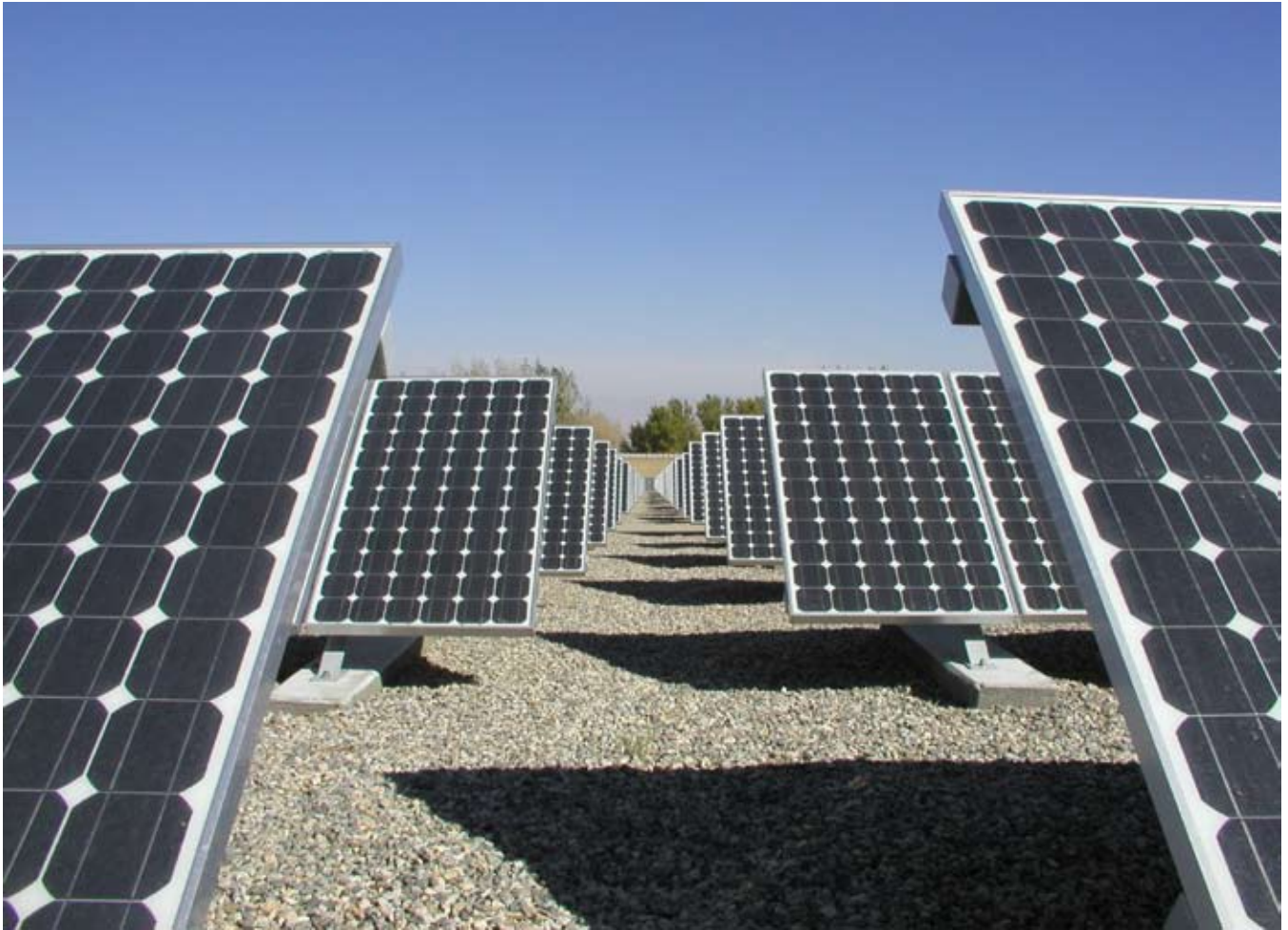
One megawatt solar field at Cerro Coso Community College's Ridgecrest location in California.
